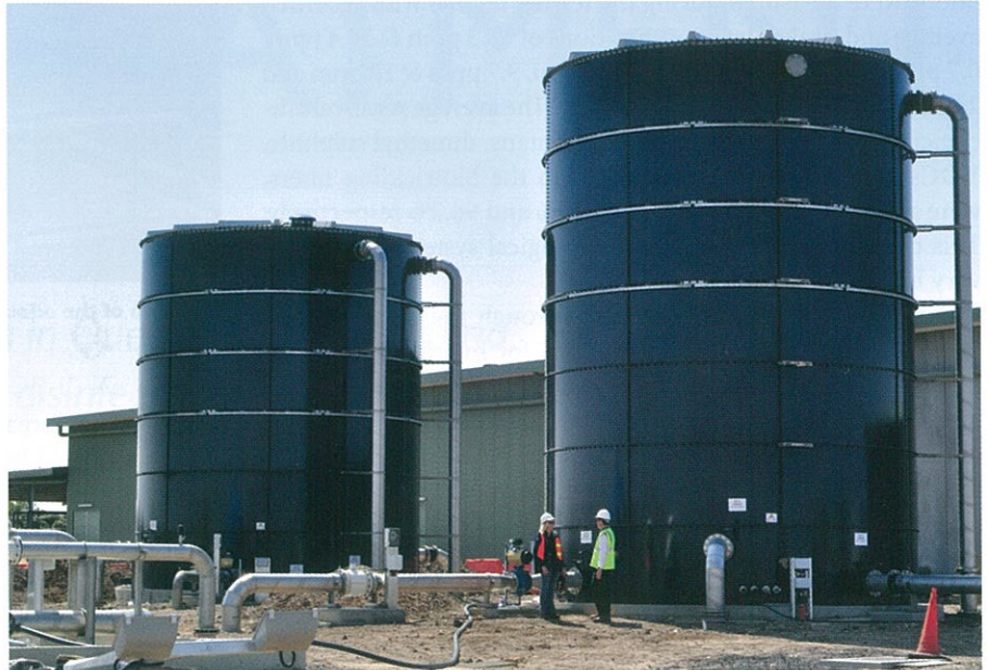
The Black Rock Recycled Water Plant will produce Class A water for housing developments and Class C water for agriculture and recreation.
